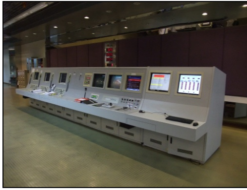
Fig. 9 - Remote Monitoring Computer at Central Control Room
